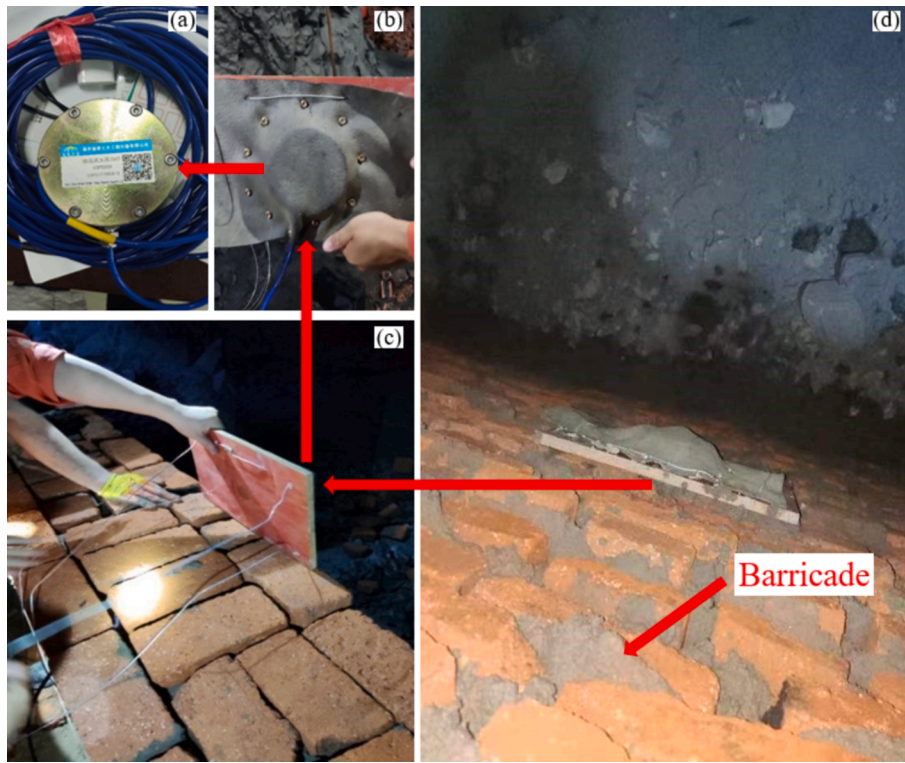
Fig. 4. Sensor installation process. (a) Earth pressure sensor; (b) Processing of the sensor; (c) Fixing of the sensor in the barricade; (d) Completion of the sensor installation.
