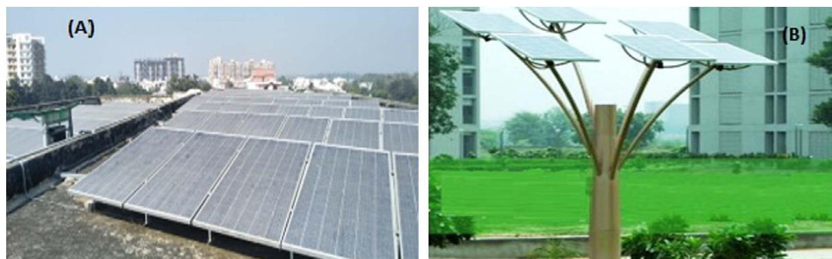
Figure 3. A classic PV rooftop power plant of 20 kW capacity installed in a large land area (A) and a SPVT of 20 kW installed in a small land area (B).
