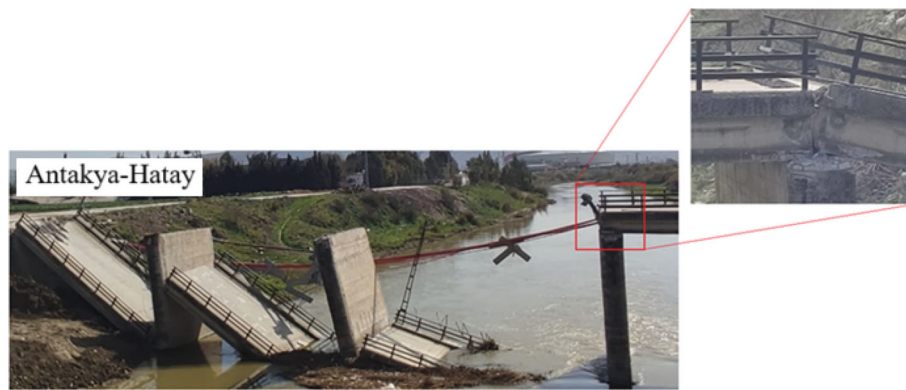
Fig. 1 Partially damaged bridge due to ground failure during February 6, 2023, Kahramanmaraş earthquakes in Turkiye
